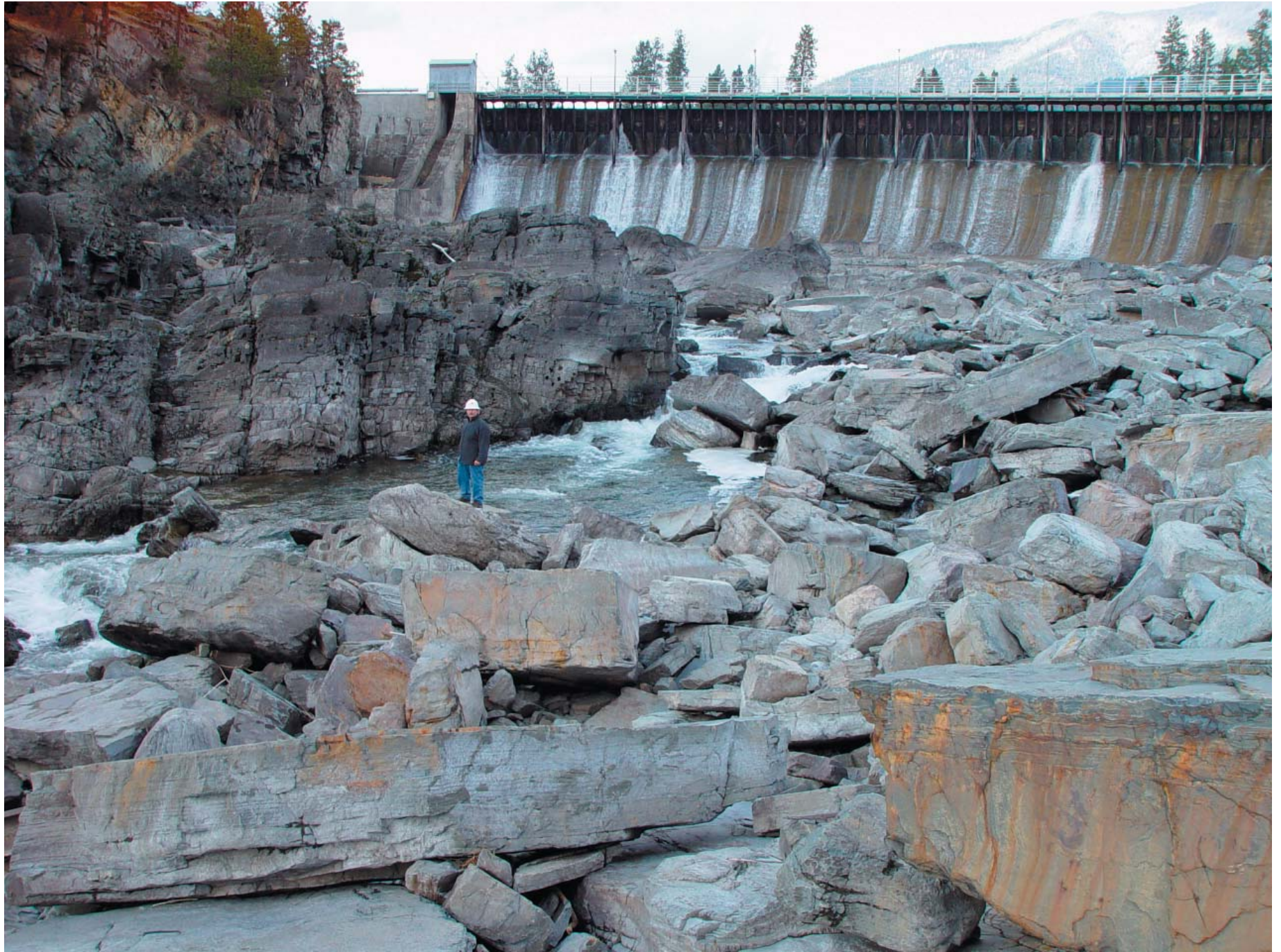
Main Dam Spillway - Spillgate Leakage Only
